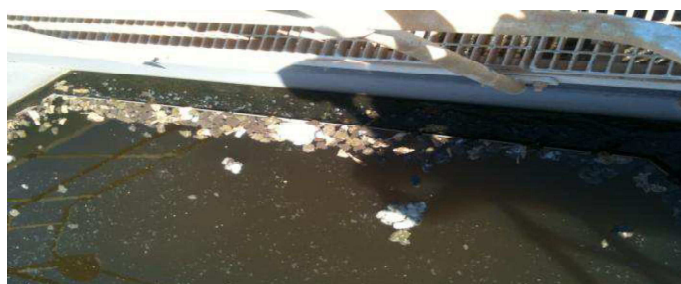
Fig.2 : photo of aeration chamber
