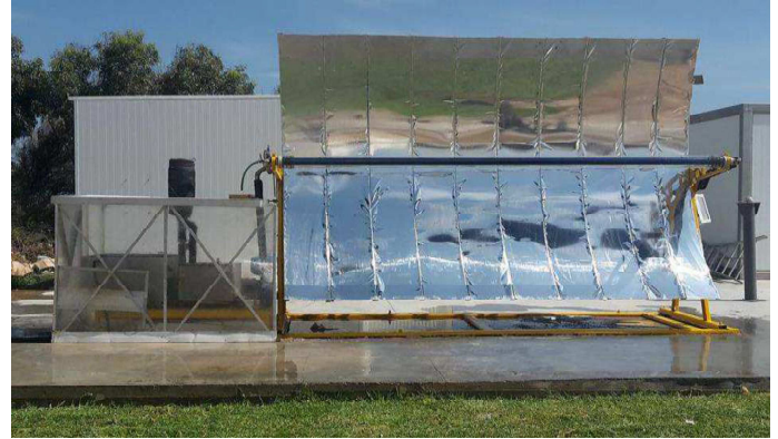
Fig.1 Real image of Parabolic Trough Collector in CRTEn
